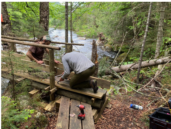
Repairing Elevator Shaft bridge after a large spruce tree fell on it
